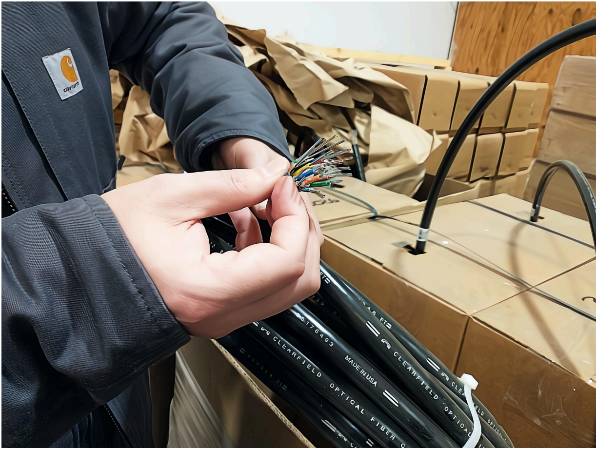
Tom Innes from APB shows the individual fiber strands contained in a distribution cable. These cables will connect the cabinets together, with smaller and lighter cables running to homes.
