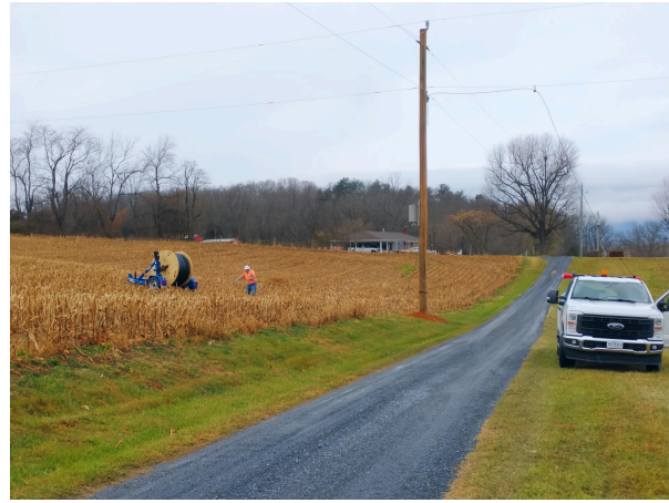
Two new poles were installed by Dominion for this area, replacing aging poles that were substandard and not suitable for carrying fiber optic cable.
