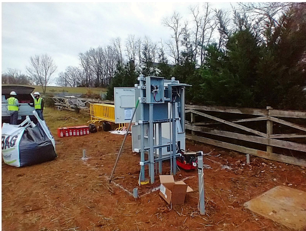
The electric service from Dominion will be installed in the gray box in the foreground. In the left background can be seen the backup batteries for continuous service. A small concrete pad for the emergency power generator can be seen on the ground to the right.
