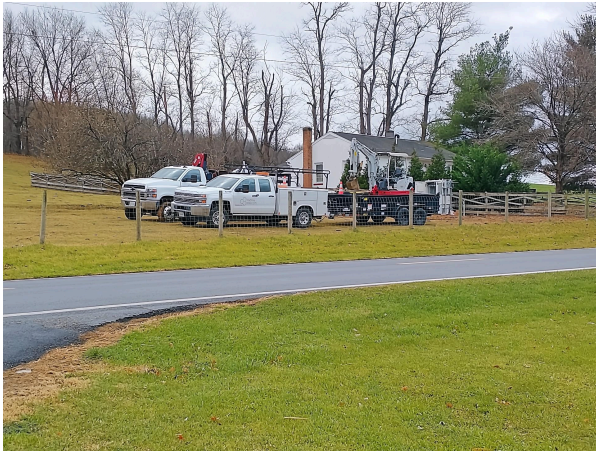
The active cabinet is located along a main road, but is on property outside of the VDOT right of way (ROW) for the road. APB contracts with property owners for lease agreements to host the cabinets on their private land.
