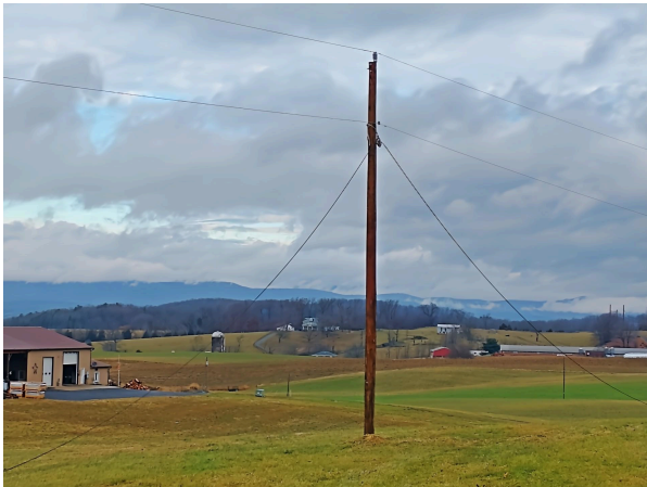
One of the new poles installed by Dominion, which will carry the cable back to the active cabinet for service to these homes.
